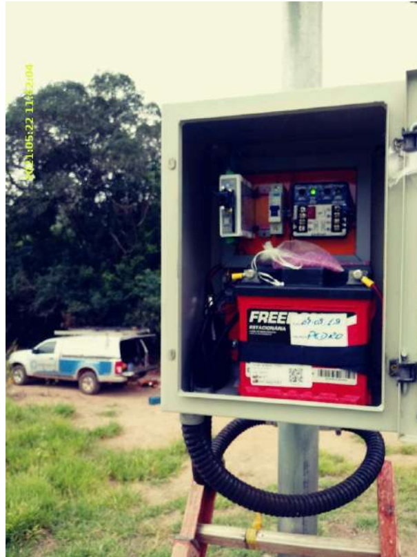
Interior do Painel
