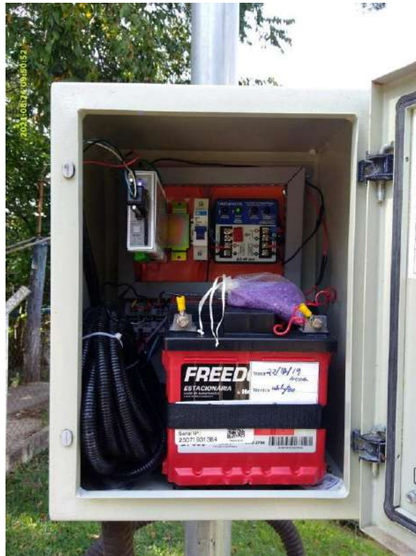
Interior do Painel
