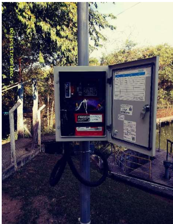
Interior do Painel
